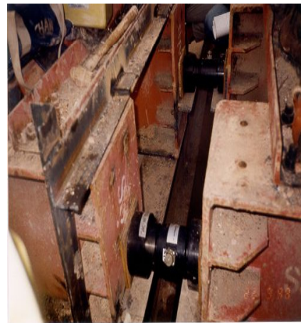
A typical load cell installation
