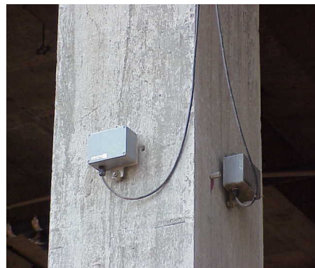
EL Tiltmeter installed on column
